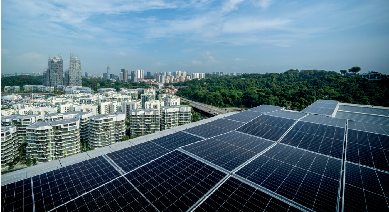
Photovoltaic panels installed on the roofs of Keppel Bay Tower and its six-storey podium block generate an energy yield of about 100,000 kWh per annum to power the building.
